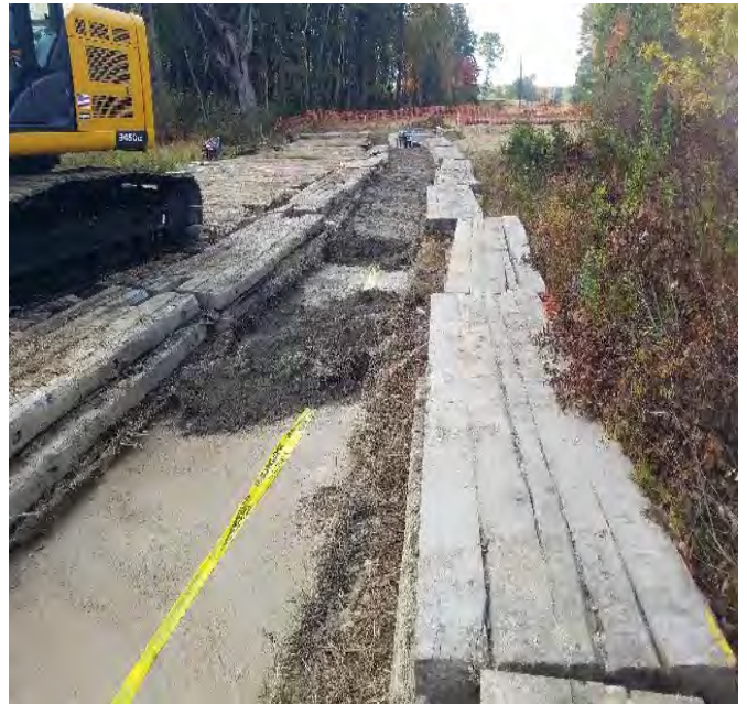
Fig 10: Restoration of trench through wetland NW16 on the Frink farm. Viewing west. (10-14-19).
