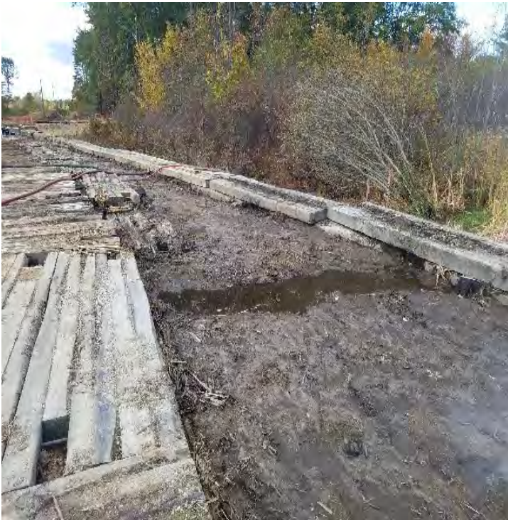
Fig 31: Rain water accumulation in Knights Brook restoration at Frink farm. Viewing west. (10-18-19).
