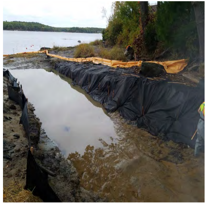
Fig 6: Bank stabilization in trench on the east side of the Bay. Viewing west. (10-12-19).
