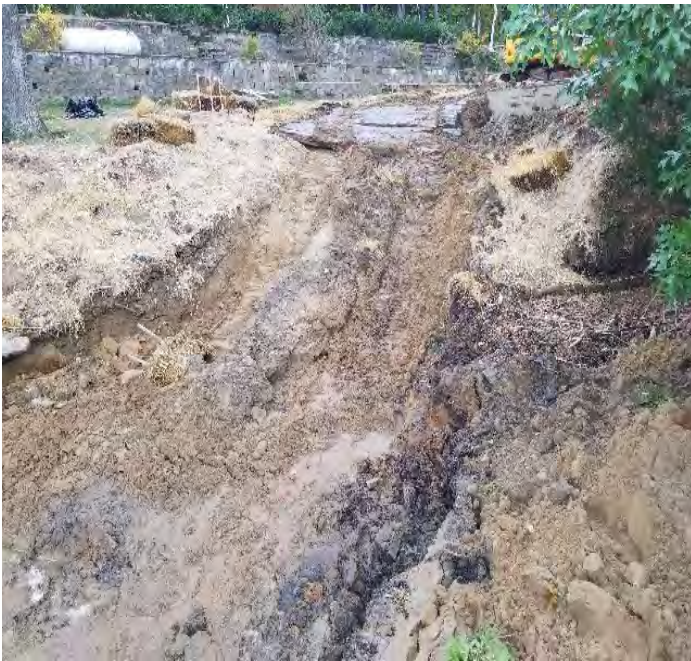
Fig 3: Blu Rock began trenching activities in intertidal zone at Beswick property. Viewing northeast (10-11-19).
