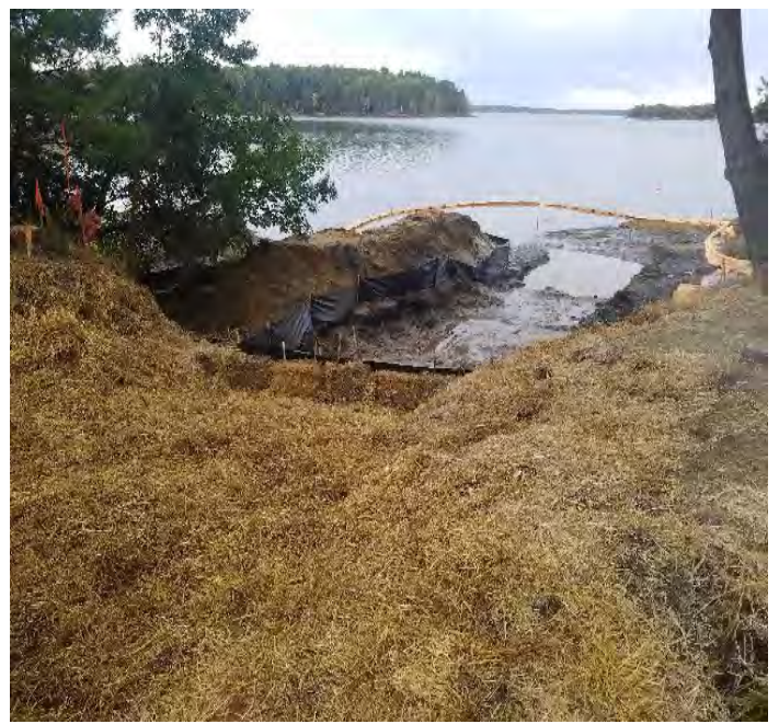
Fig 4: Sediment controls installed on the east side of the Bay. Viewing west. (10-11-19).
