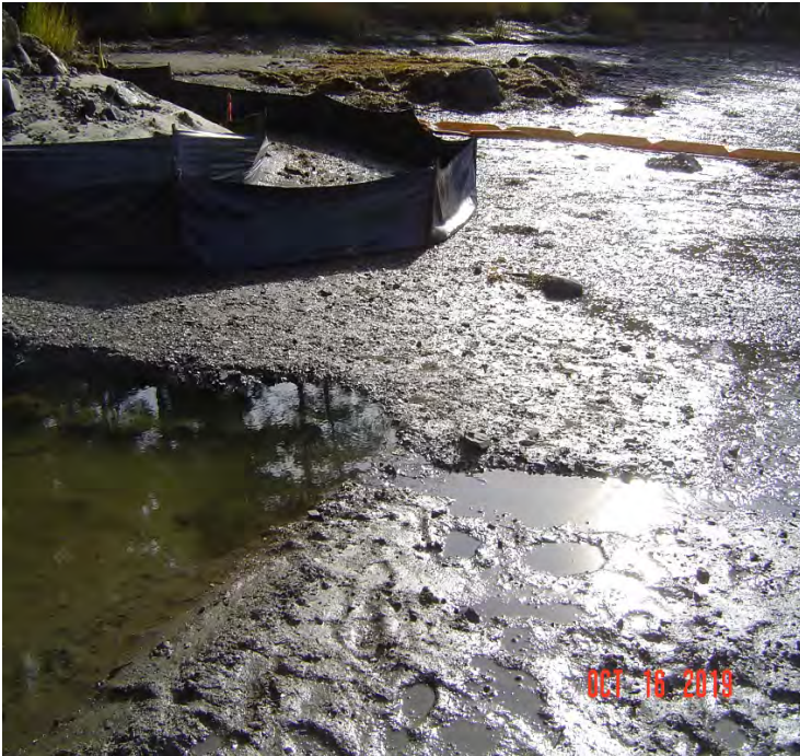
Fig 25: Sediment controls in intertidal zone on the east side of the Bay.
